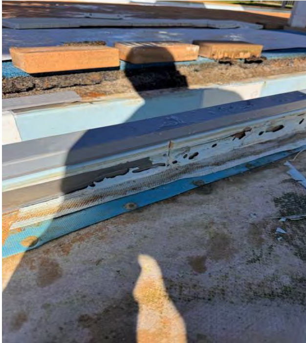
No Geotextile on ramp.
